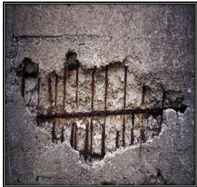
Figure 47 Corrosion in Concrete
