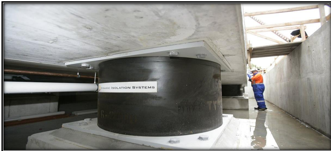
Figure 70 Base isolation system
