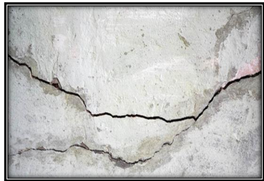
Figure 48 Cracks in concrete
